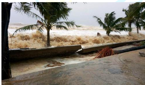
Photo: Dam and sea embankment in Thanh Hoa are broken by Typhoon No. 10
