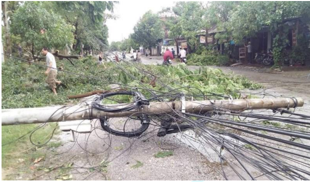
Photo: Electricity pole broke down due to Typhoon No.2 in Ha Tinh province
