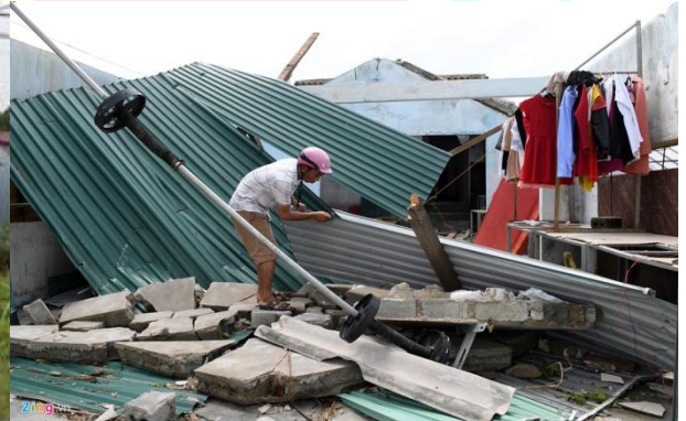
Photo: House damaged, roof blown off due to Typhoon No. 10 (Doksuri) in Ky Anh, Ha Tinh province
